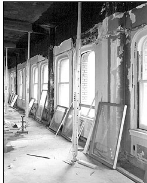
The Cobb's large, operable windows allow natural light and ventilation. Low-e film was applied to the glass to improve thermal insulation.
