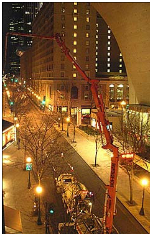
Most concrete work was done at night so that tenants were not interrupted. Concrete was pumped through 250 feet of hose from Fifth Avenue.
